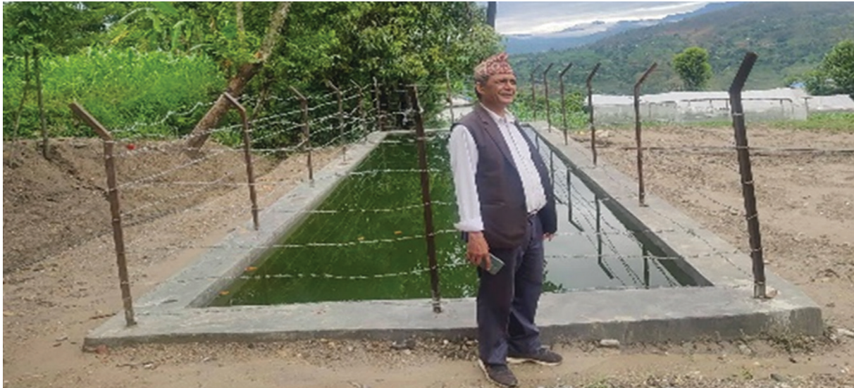
Figure 9: Chairperson of Kritidewal Cooperative of Narayan Municipality posing by the newly constructed collection pond.
